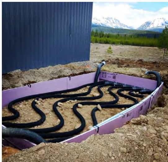
The two-foot layer of perforated piping and insulation in a passive system. Photo: Dave McC Carson
