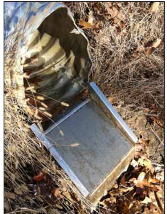
The intake can use an existing conduit – a road culvert in this case. Photo: Leif Kindberg, NCAT
